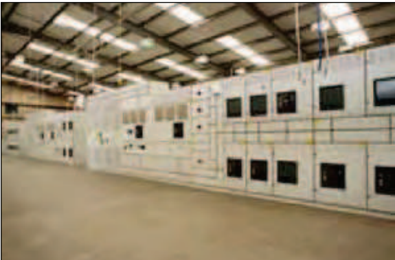
6300A Package Sub Station
